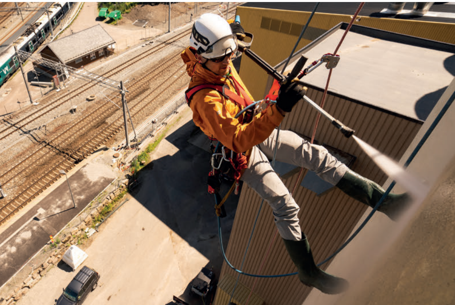
Torbjørn Solheim carrying out high pressure cleaning operations on the Felleskjøpet building. Torbjørn Solheim realiza tareas de lavado a alta presión en el edificio de Felleskjøpet. Eidsvoll, Norway (courtesy of Varri AS, ph.Kyrre Buxrud).
